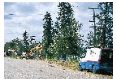
In 1994 Telecom Finland installed 2,500 km of fibre optic cable, bringing the nationwide total to 13,000 km of optical cables containing 160,000 km of optical fibre.
