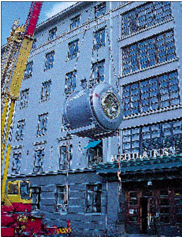
The Christian Nissen Department delivered to the X-ray Department of the Meilähti hospital a Picker Edge 1.5 T high field magnet equipped with state-of-the-art accessories. The magnet, hanging from a crane, was handily lifted to the sixth floor by way of a hole made in the roof. The unit weighs about 7,000 kg.
