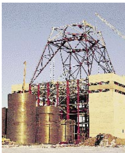
Construction of a large-scale power plant in St Petersburg began in early 1995.
