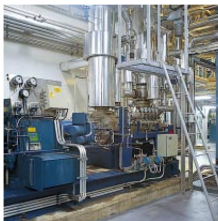
Several different types of pumps and valves were supplied to the back-pressure power plant of the Rovaniemi Power Utility.
