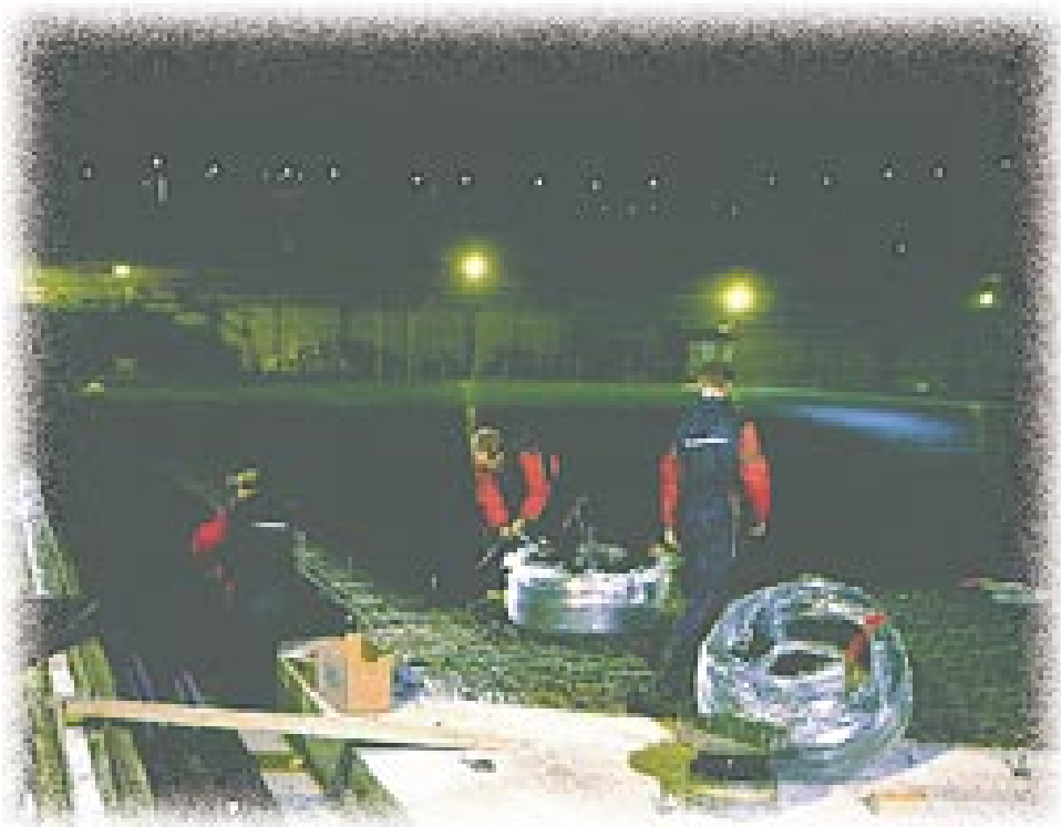
Uponor Finland supplied some 25 kilometres of PELM-pipes for cooling the rink of Helsinki's new Hartwall Arena, venue for the 1997 World Ice-hockey Championships.
