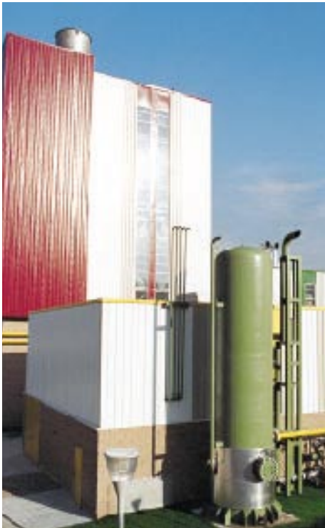
Enso Española's combined-cycle power plant near Barcelona was started up in autumn 1996. Ekono Energy's services for the project included engineering, supervision and procurement.
