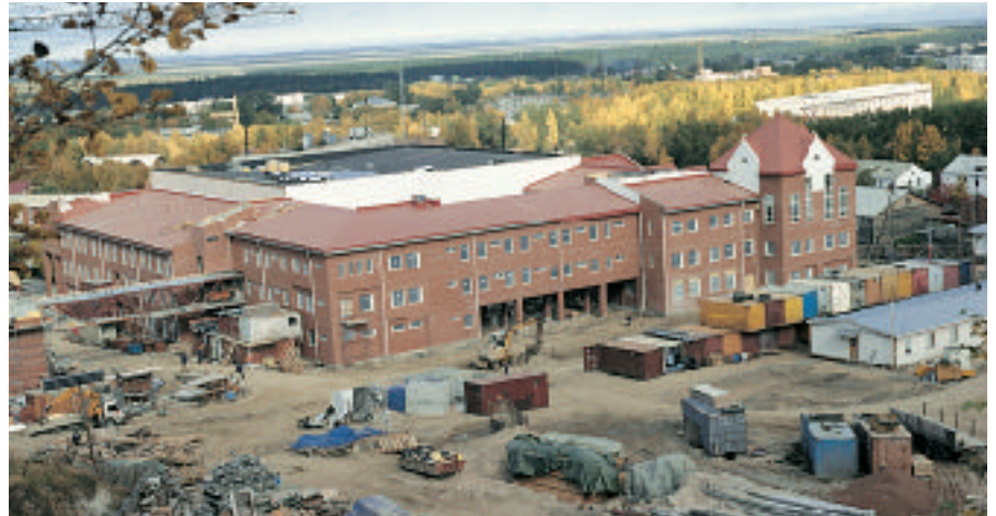
Lemminkäinen Construction's largest overseas project was an art school and cultural centre at Khanti-Mansiisk in Siberia.
