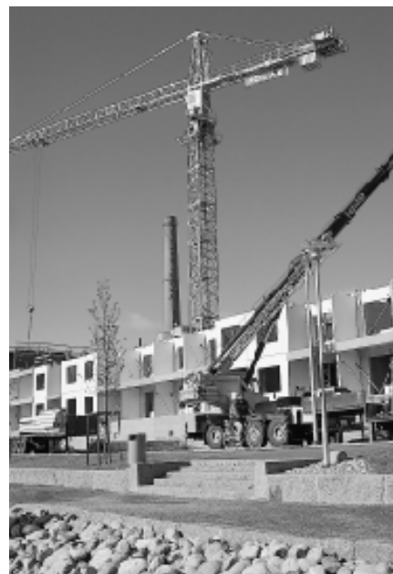
The photo shows a rental apartment unit built by Polar's Western Finland unit for the Local Government Pensions Institution on the Aurajoki river front in Turku. The development will have 119 apartments and 129 parking places.
