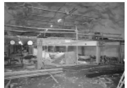
In addition to extending the underground car park in the Kamppi district of Helsinki, Polar is building an underpass from the Forum mall's underground car park to the Sokos department store.
