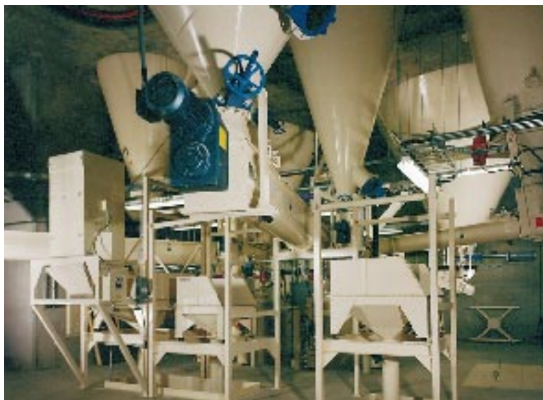
Receiving and dosing equipment for minor ingredients at Guardian's Bath Plant.
