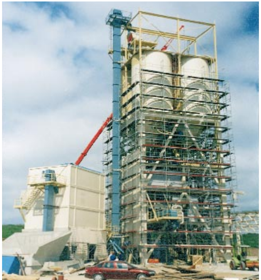
The plaster and mortar plant delivered to Rethwisch Baustoffwerke in Germany was Raute Dry Mix Oy's biggest project during the year 1996. The photo shows the plant under construction.
