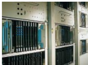
Base station controls and transcoder based on GSM/DCS voice coding at Siemens' test centre.
