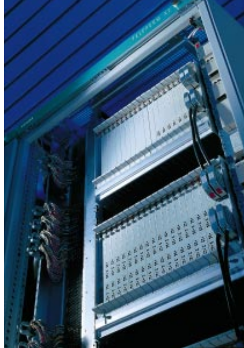
Teleperm X represents the latest power plant automation technology.
