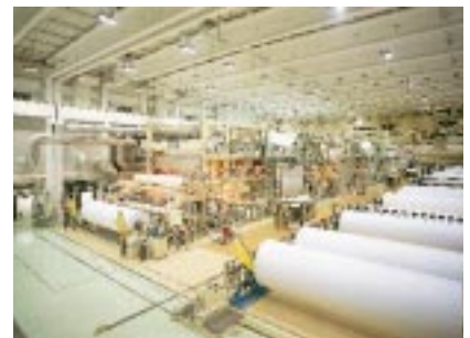
An off-machine coater with four AutoBlade coating heads on the art printing paper line at UPM-Kymmene's Nordland Papier mill in Germany.
