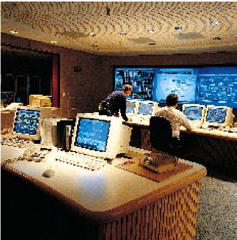
OASyS open architecture information management systems have captured more than 50 % of North American markets for oil and gas pipeline transit control. The photo shows the control room of the Kern River Company's gas line in Utah, USA.
