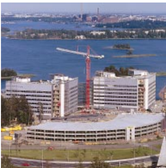
YIT carried out the construction of the Nokia House in Keilalahti as a project management contract for Nokia Corporation, Espoo.
