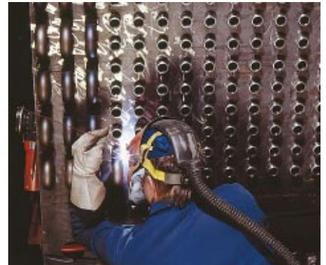
YIT Huber delivered a total of about 80 kilometres of piping, including installations, for stock handling and pipe bridges within the framework of the Fibre 90 project at the new Kaukas pulp mill of UPM-Kymmene Oy in Lappeenranta. The delivery furthermore included, among other things, the installation of more than 4,000 hand-operated valves as well as pulp and storage tanks.
