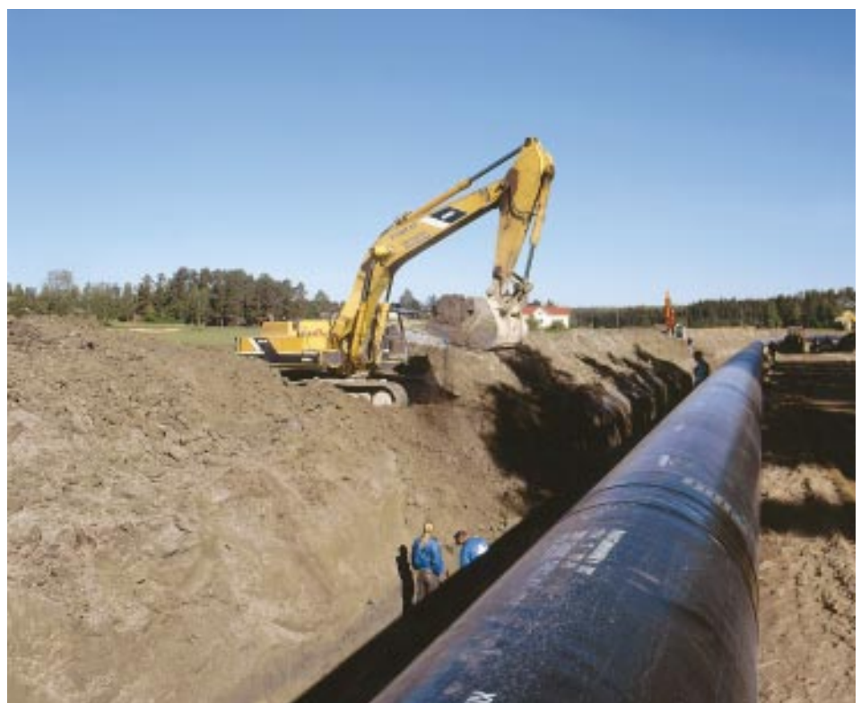
One of the major projects during the year was the building of the 48 km parallel pipeline - 900 millimetres in diameter - for the natural gas main pipeline on the stretch Imatra-Törölä for Gasum Oy.
