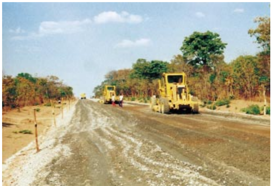
Work started on a highway improvement contract covering a 200-kilometer stretch of road in Zambia.
