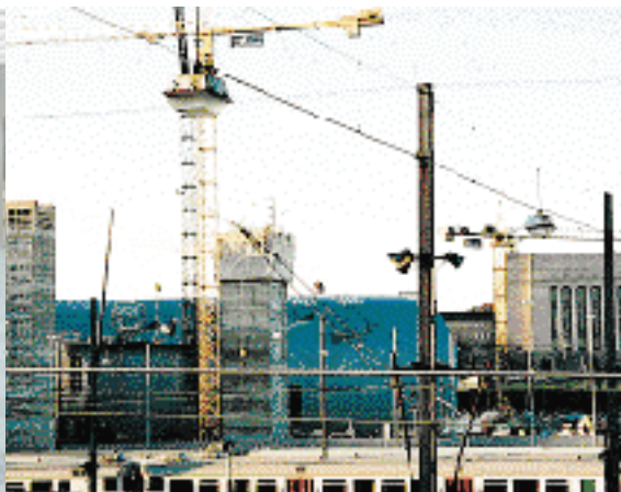
The frame for the Sanoma Oy newspaper house will be cast in situ on the plot next to the Kiasma building in the centre of Helsinki.
