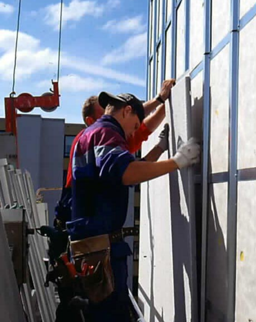
Renovation of an apartment building facade. Rannila's Liberta cassette panels are used as the wall cladding.
