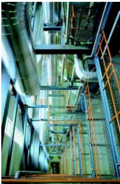
SCA Mönsterås, recovery boiler, Sweden.
