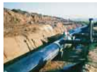
Maghreb-Europe gas pipeline, Spanish section
