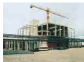
CMC-plant, Metsa Specialty Chemicals, Finland
