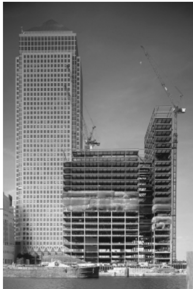
CitiBank's 27-story European headquarters in London is being built by Canary Wharf Developments. KONE is supplying 12 KONE 9000 scenic elevators to the building. The main contractor for the project is Bovis/LEHR McGovern.
