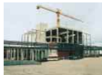
CMC-laitos, Metsa Specialty Chemicals
