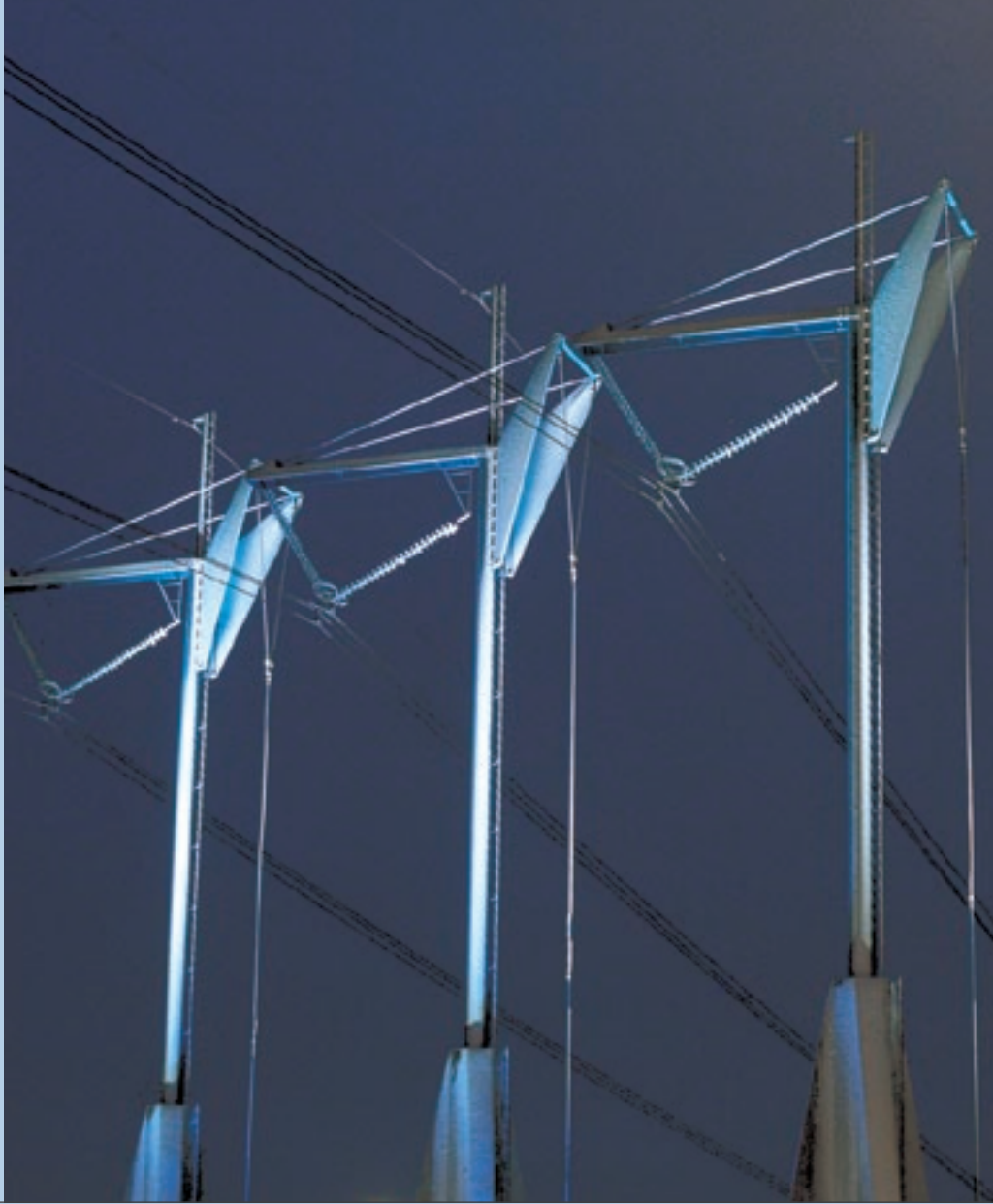
The environment and power transmission – Ensto's power line accessories on an eco-pylon belonging to Suomen Kantaverkko Oyj, the national network operator.
