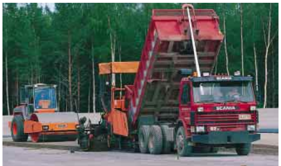
An extension to the Rusko landfill in Oulu was built using a watertight asphalt structure. Mineral insulation work in progress.
