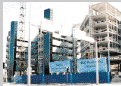
The appearance of work sites is clear and in line with the company's graphical line.
