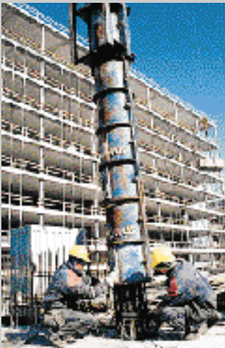
The general orderliness of a building site guarantees working safety and free-flowing information ensures smooth working.
