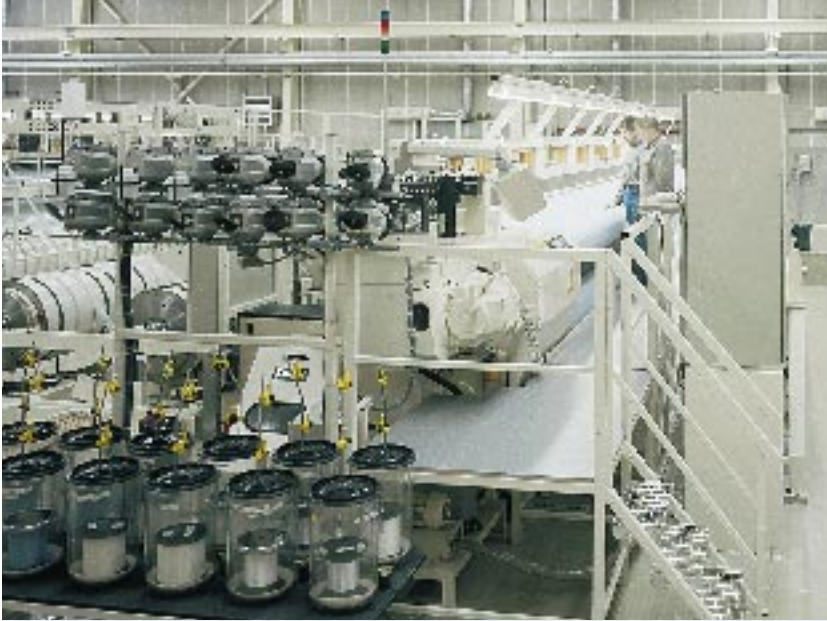
A new 13.5 m wide Jäger loom at Juankoski enables Tamfelt to supply clothing for the world's widest paper machines.
