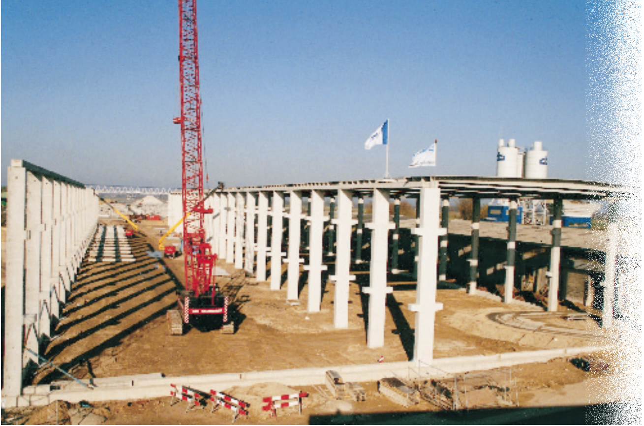
Growing popularity of hollow-core slabs demands additional manufacturing capacity. The subsidiary Spanbeton provided the factory frame for the new VBI plant.
