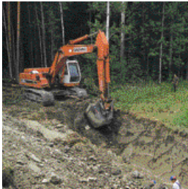
The parallel pipeline from the Imatra reception station heading towards the parallel pipeline under construction in the Karelian Isthmus crossed the Finnish-Russian frontier in July, under the watchful eyes of frontier guards.
