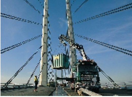
The 8 km Öresund Bridge is one of the longest in Europe. Hiab loader cranes, which have been used extensively throughout the bridge's entire construction, perform demanding lifting of site cabins, steel components, machinery and waste containers.
