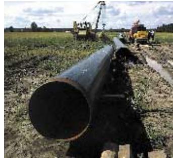
PVO is a member of a Nordic consortium investigating the prospects for constructing a natural gas pipeline from Haltenbanken in Norway through Central Sweden to the west coast of Finland. The aim is to construct a gas network supplying the west coast, which will later be linked to a gas pipeline from Russia.
