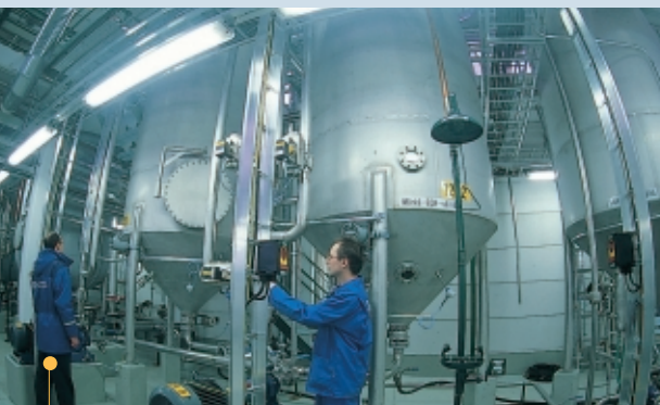
The Raisio Chemicals plant in Mietoinen produces cationic chemicals used for starch conversion. Such modification improves the binding of starch and fillers to pulp fibres in papermaking.
