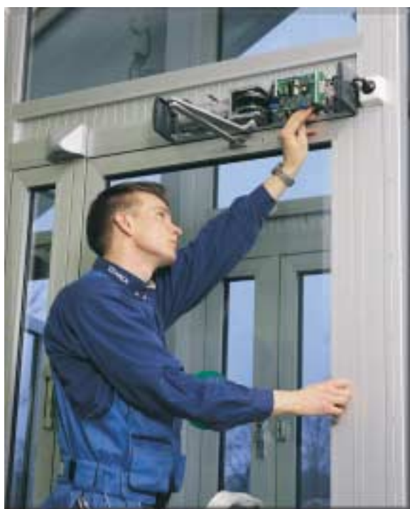
Automation is a significant part of the door-system functionality.
