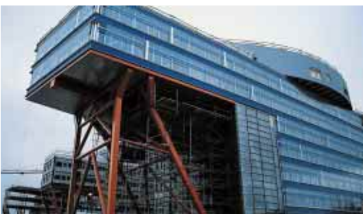
■ Plumbing and electrical works are being carried out at the High Tech Center in Ruoholahti, Helsinki.
