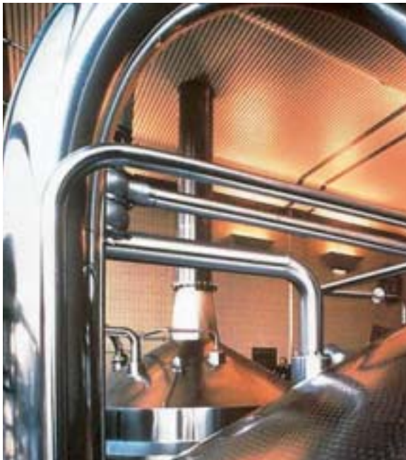
The food and beverage industry appreciates the hygienic properties of stainless steel.
