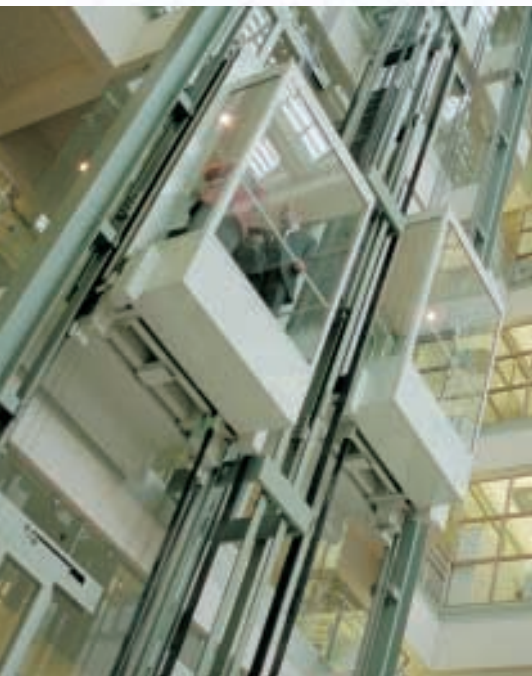
Etteplan has made numerous significant partnership agreements. Among its important partners is Kone Corporation, to which Etteplan provides lift R&D and design services. (Photo: Kone)
