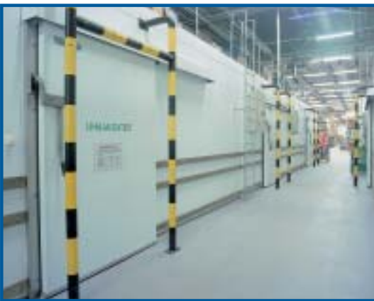
Cold rooms in the shopping mall, Mylly, Raisio, Finland.
