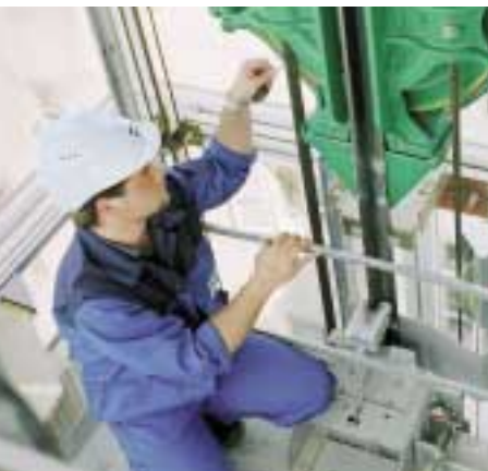
KONE is a global service company and technological leader in its field. Innovative products and maintenance services based on the latest technology guarantee efficiency and create added value for KONE customers.
