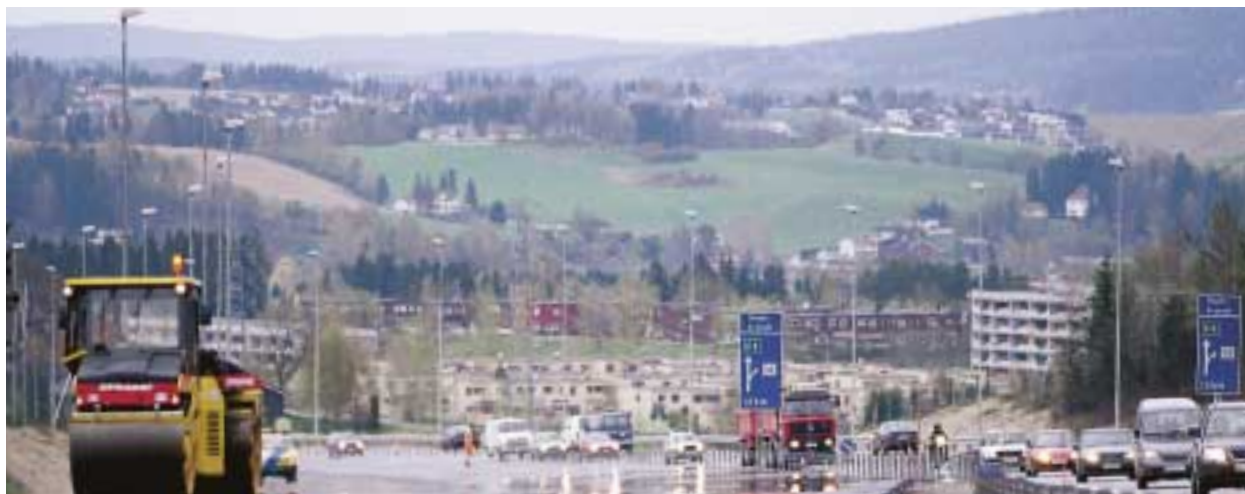
Lemminkäinen has about 17 % share of the Norwegian asphalt paving market. Paving work in progress on Highway E6 near Oslo.
