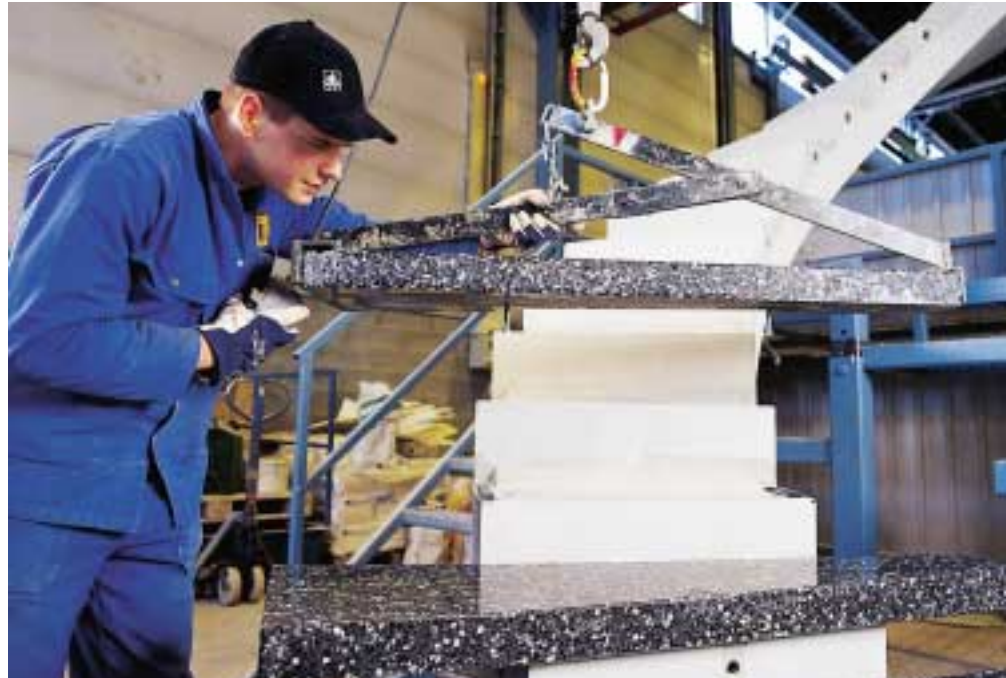
Lemminkäinen has been manufacturing stairs for over 90 years. Ville Tuunanen assembling a precast stair unit.
