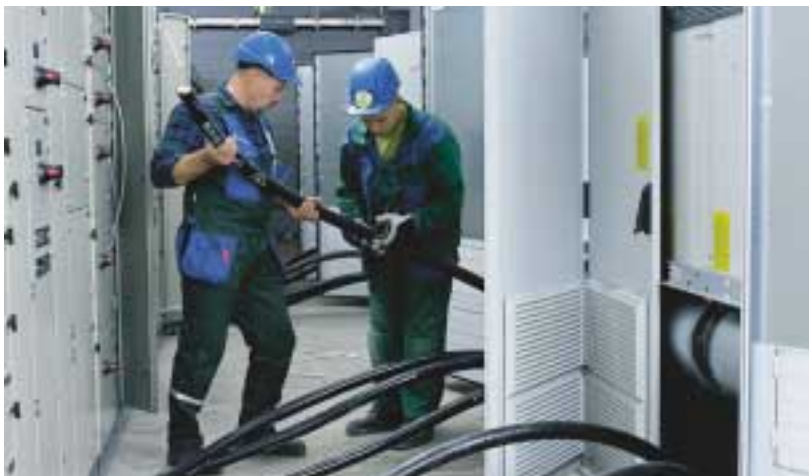
Boiler electrification and instrumentation works were carried out for Jämsänkosken Voima Oy.
