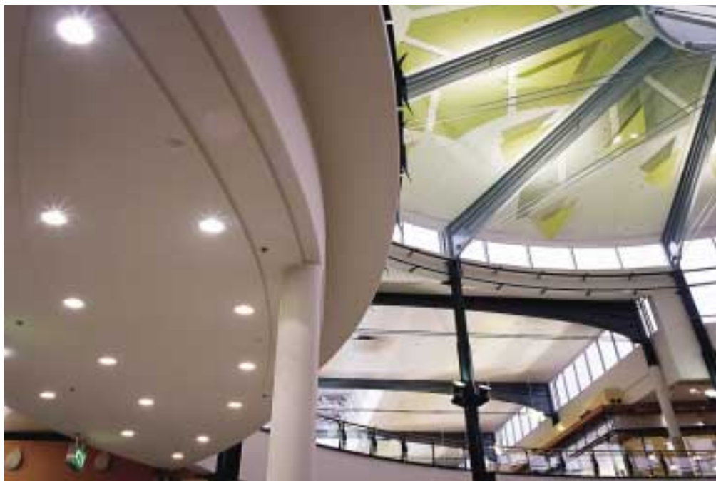
Tekmanni supplied the sprinkler system for the Mylly shopping centre in Raisio. The company also carried out the building's electrical contract.
