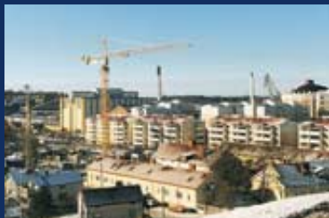
In Turku, a sheltered housing facility is under construction. It will feature communal apartments, a service centre and a daycare facility.
