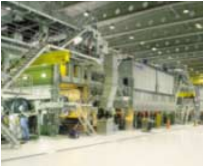
Continuous monitoring of moisture in a paper machine's lubrication system helps prevent breakdowns and unscheduled downtime.
