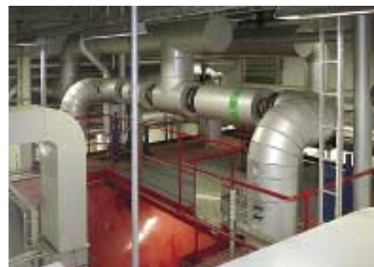
Total installation of SAAB Trollhättan's oil boilers.
