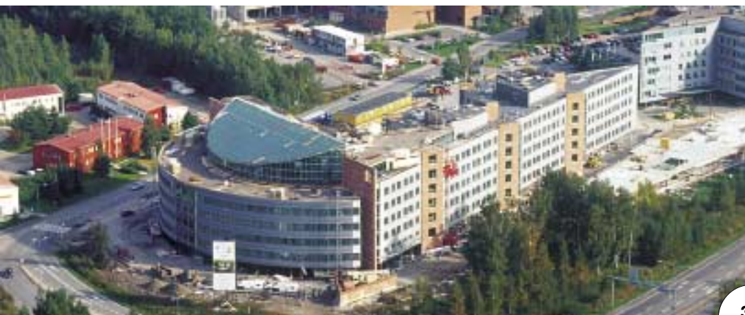
The Innopoli II site's victory in the Construction Site of the Year 2001 competition is evidence that the development of work site management methods and culture has brought results.
