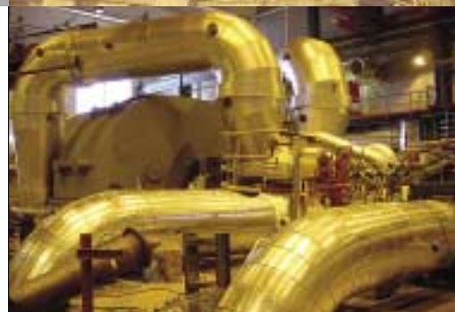
The turbine hall of the Alholmens bio-energy plant. YIT was responsible for the design, manufacture and installation of the high- and low-pressure piping.
