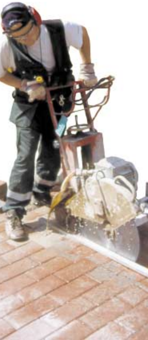
YIT Rapido carried out the yard works of the Leppävaara health care centre.
