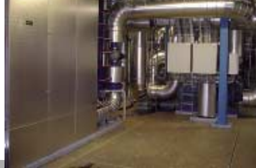
Distribution pumps of the Kumla district-heating centre.
