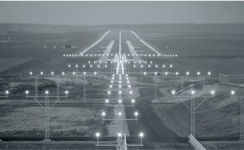
Exel delivered 200 approach light masts to Helsinki-Vantaa Airport's third runway.
