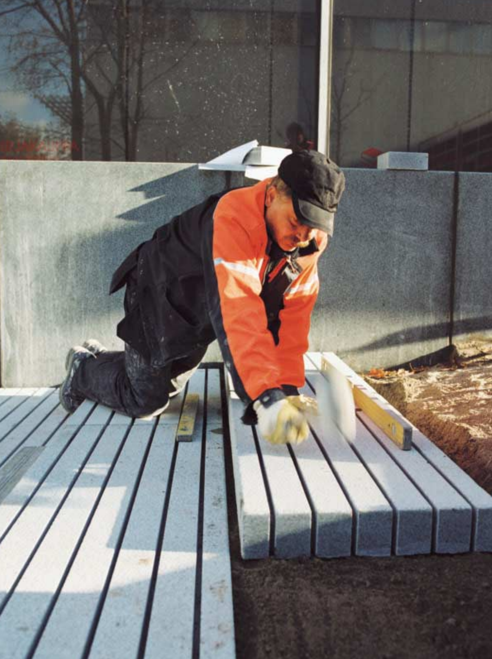
Stonemason Jari Sirén installs granite steps on site in the centre of Tapiola.
