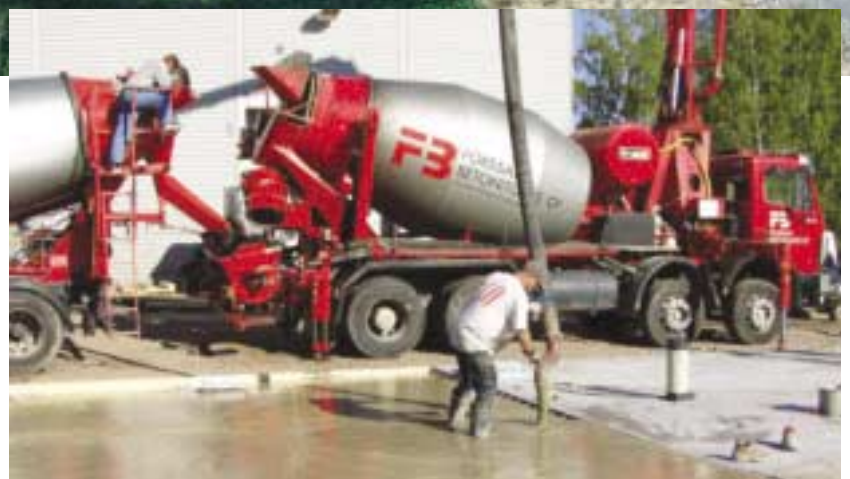
Floor concretes have been one area of Forssan Betonituote's product development work. The photo shows a warehouse floor being laid in Talma, Sipoo.
