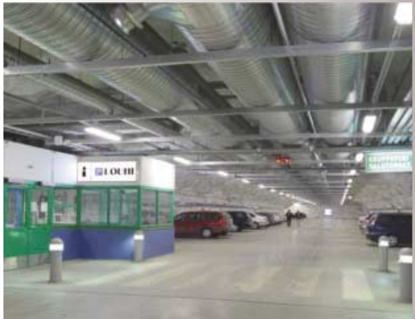
Tekmanni made the HVACE and sprinkler installations in the P-Louhi underground parking facility in Turku.
