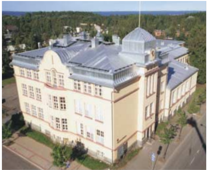
The renewal of the Joensuu Workers Institute's multiform metal roof, which Lemminkäinen carried out in 2002, was highly commended by the Finnish Roofing Association in connection with its Roof of the Year competition.
