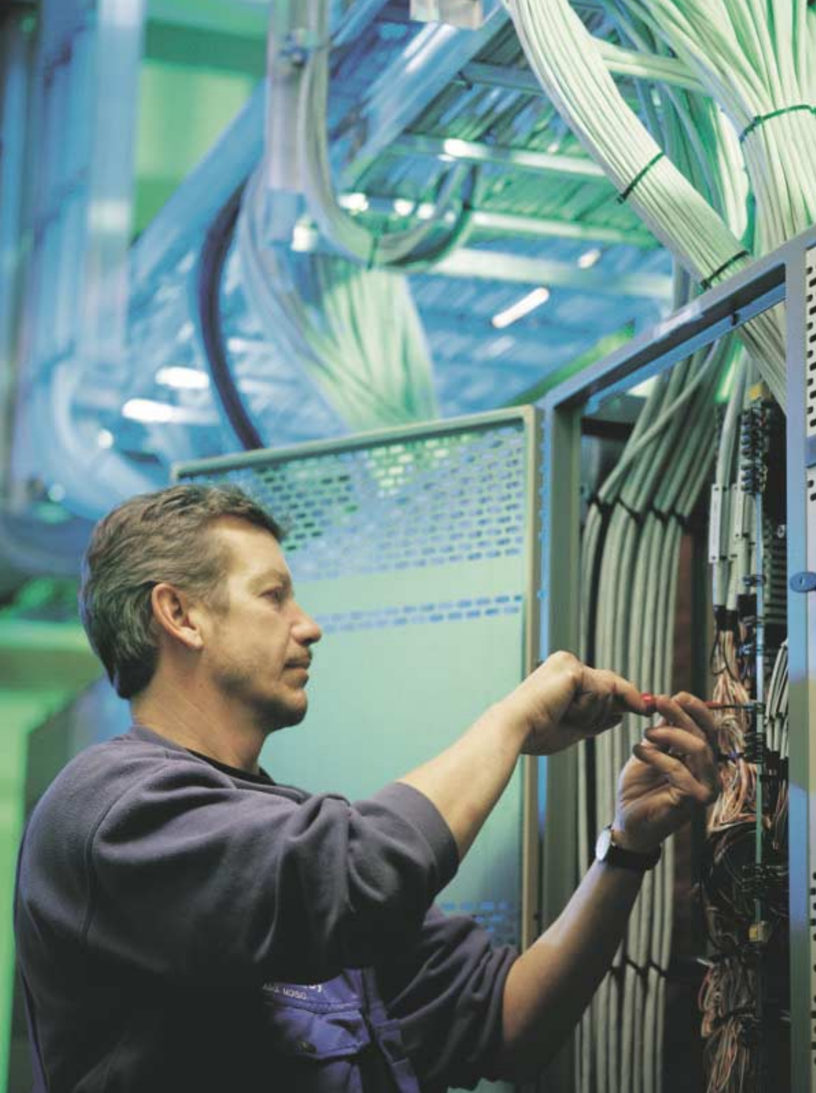
Fitter Juha Moisio connects cables to the automation system at Äänevoima Oy's biopower plant in Äänekoski, where Tekmanni carried out the boiler plant's process electrification work.
