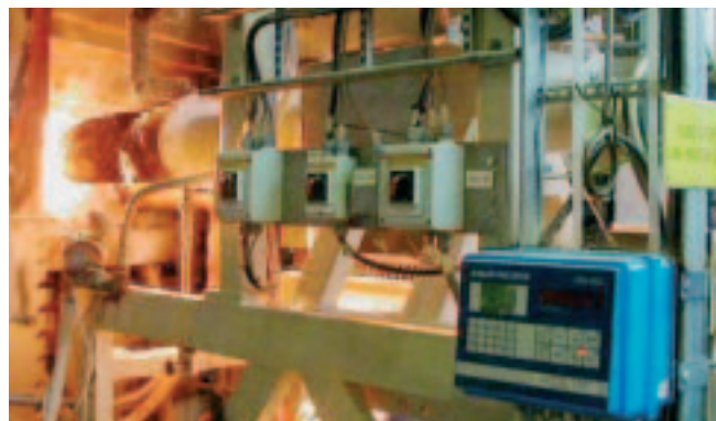
The waste fiber recycling process, developed by Raute Precision for the fiberglass industry, reduces the consumption of energy and the amount of difficult fiber waste, also improving the raw material yield.
