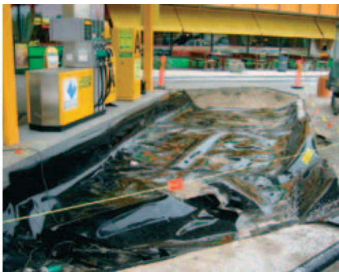
In October, plastic film was installed in the petrol pump area of Cooperative Society Hämeenmaa's ABC Karavaani to protect the soil and ground water.
