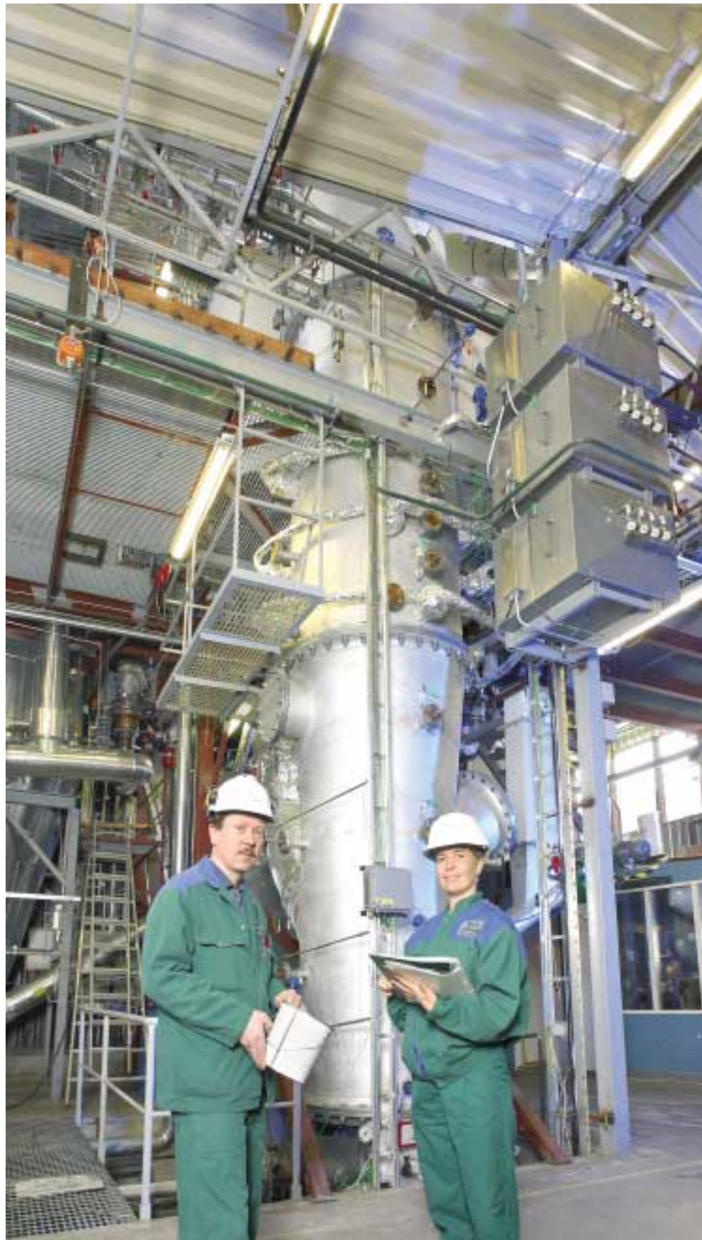
VTT's pilot plant is being used in the further development of a method whereby fuels from waste are processed into a pure gas product for combustion in large power plant boilers.
