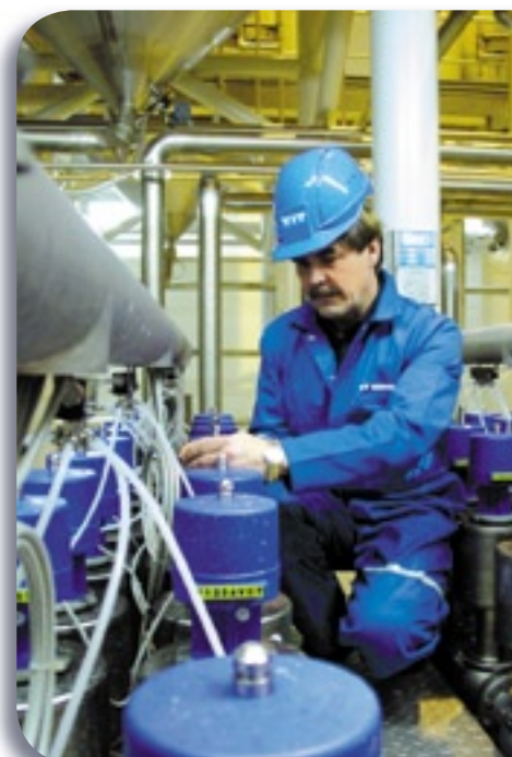
Jorma Heinonen inspecting the condition of the pump automation at Koff's factories in Kerava.
