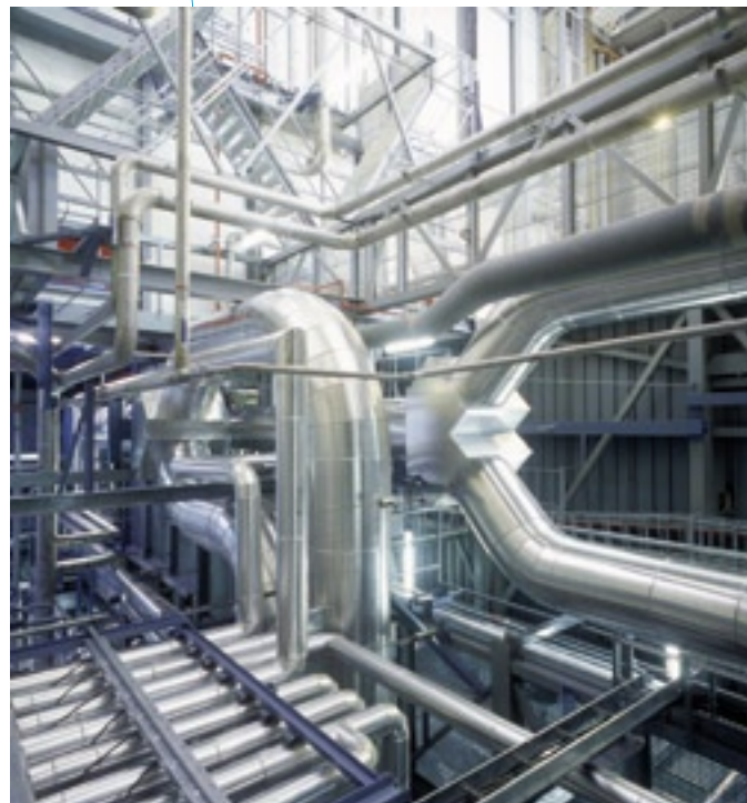
Piping of the Edenderry peat power plant, Ireland.
