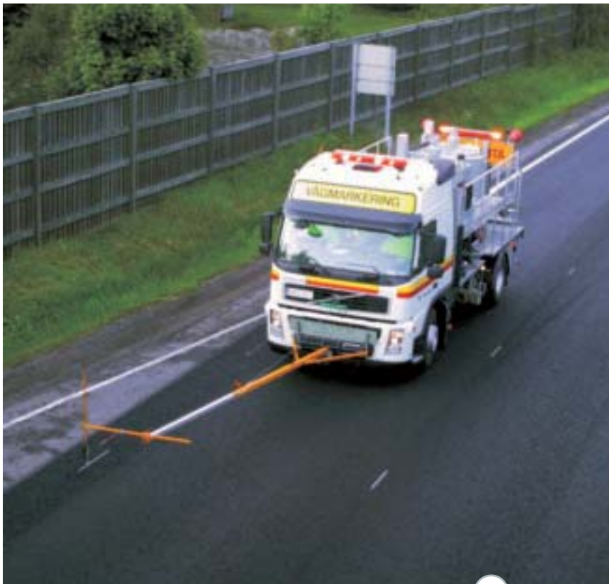
Tielinja Oy carried out road marking works in the Northern Road District of Sweden.
