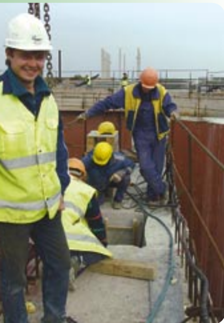
The construction of St Petersburg's southwestern wastewater treatment plant continued in 2003, carried out by SWTP Construction Oy, a company established by YIT, NCC and Skanska. The project is the most important environmental protection project to improve the state of the Gulf of Finland and the Baltic Sea.
