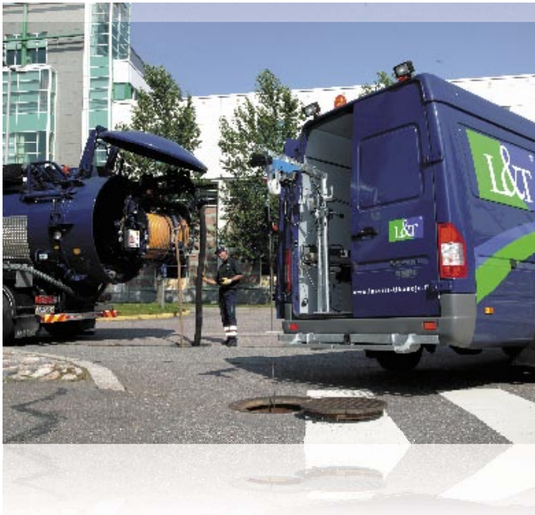
Interior camera scans reveal the condition of pipelines and locate possible damage.
