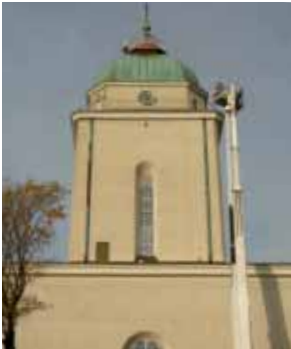
A mobile phone network base station being installed on the island of Suomenlinna in Helsinki.
