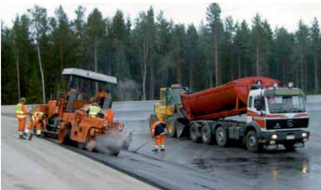
Lemminkäinen's dense asphalt pavements are well suited to soil and groundwater protection applications. A dense asphalt base being laid at the Rusko waste management facility in Oulu.
