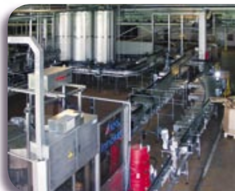
HEPAC and equipment installation works at Heineken's production plant in St Petersburg.
