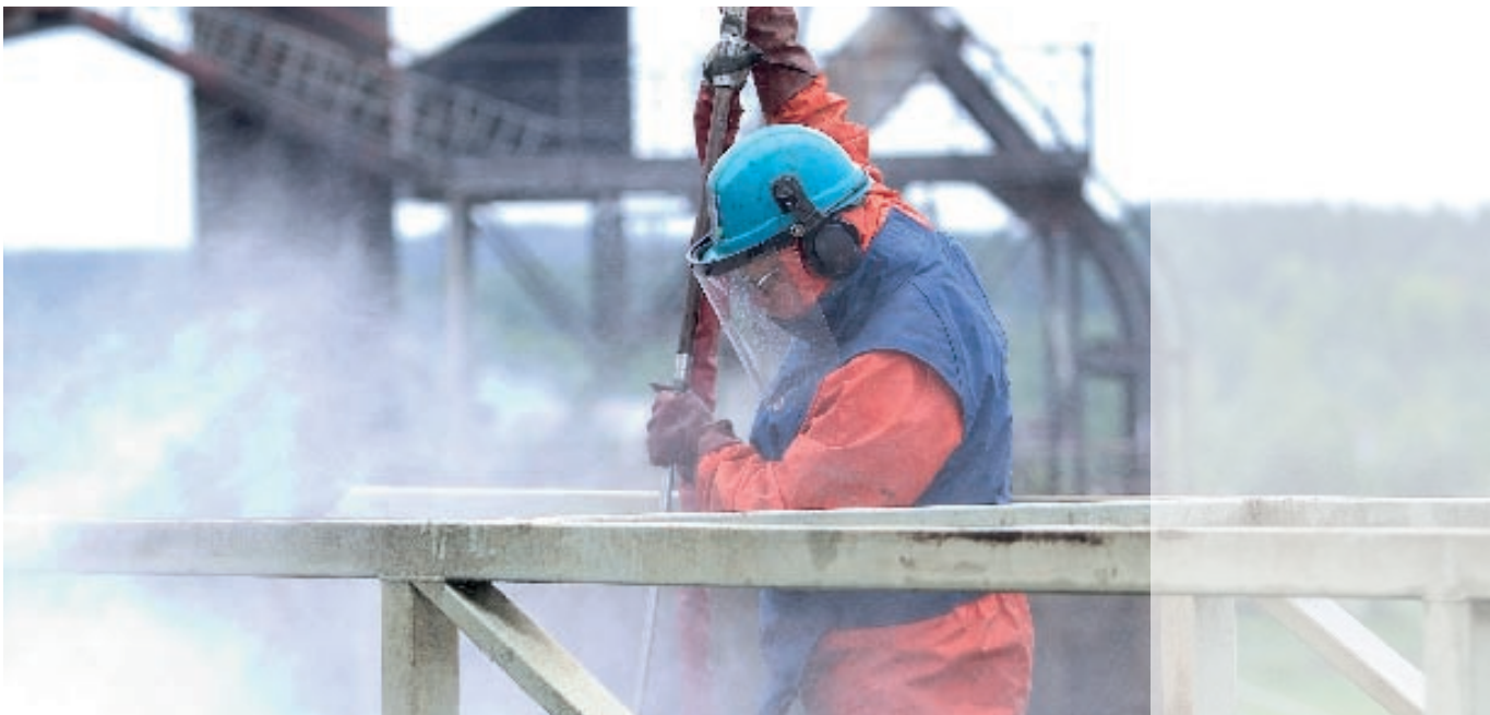
L&T's industrial cleaning services include cleaning of process pipeline systems with high-pressure water equipment.
